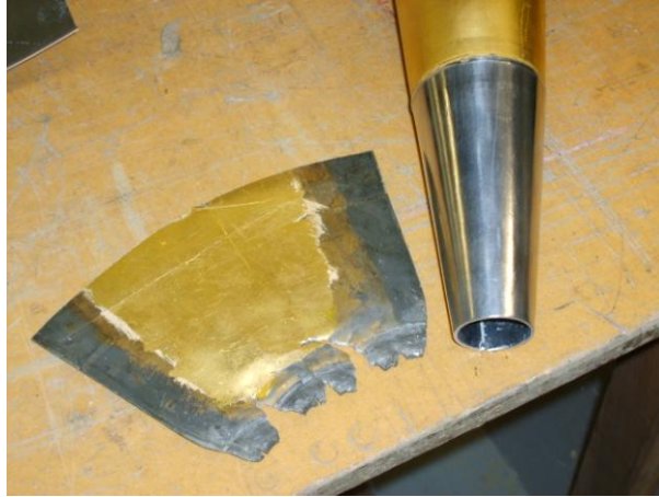
A new tip formed from the pattern of the original. With the foot now in one piece, a zinc lining can be fitted
